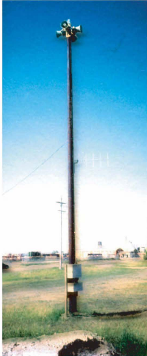
FIGURE 1 : SIREN INSTALLATION WITH STROBE LIGHT ON TOP OF THE POLE
