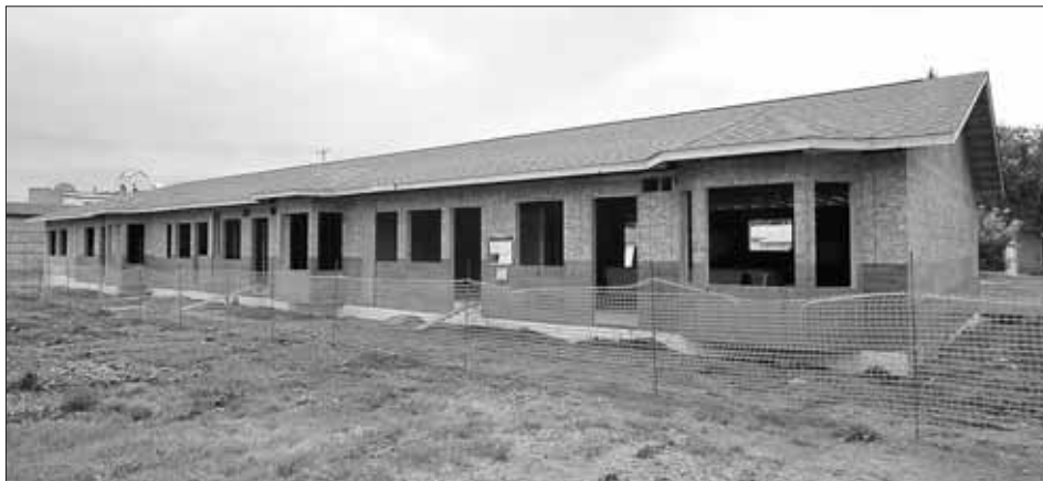
A seniors housing unit that is being constructed in Baldur. (Ed Torz/For the Sun)
