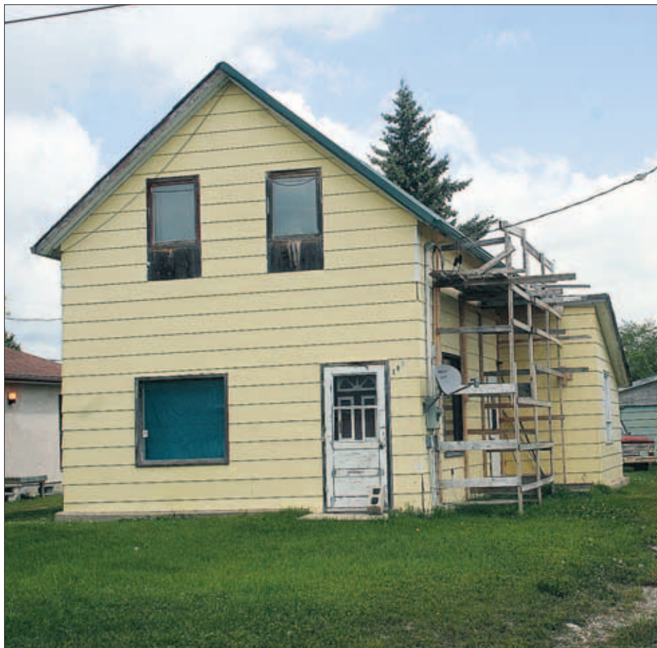
Scaffolding is set up outside a home in Minnedosa. As part of the community's 10-point comprehensive housing strategy, town council wants homeowners and landlords to consider renovating existing properties before pursuing expensive new construction projects. (Jillian Austin/Brandon Sun)
